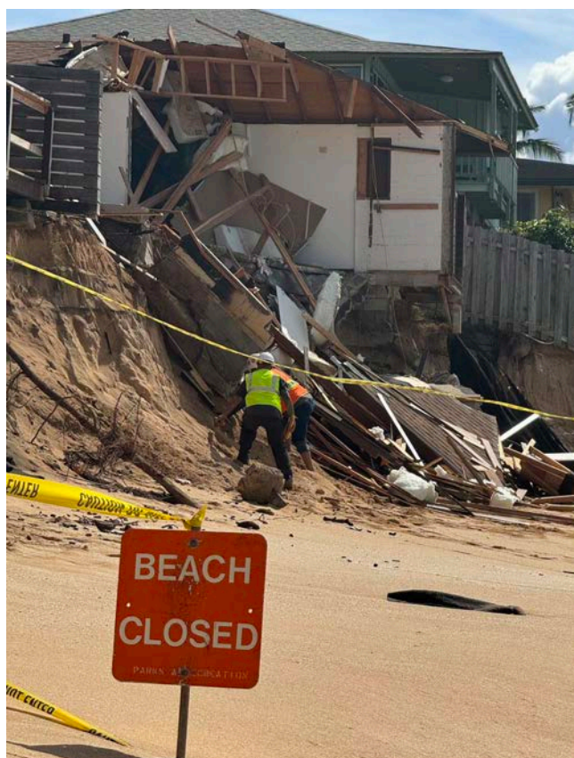
Collapsing house in the shoreline
